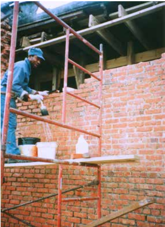
Inmate labor from Century Correctional Institute in Century, Florida, saved the Board an estimated $40,000 in renovation costs.
