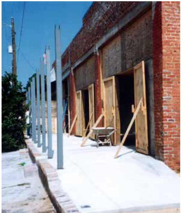
The front porch is completely rebuilt, with fresh concrete, new steps, and steel posts to hold up a new roof.
