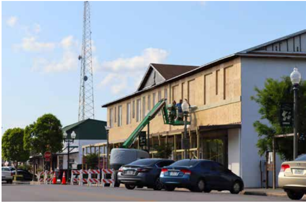
Having just removed vinyl siding, workers prepare to seal the original brickwork and windows on the Main Street façade of the former Lamar and Hilton Hotel. (Photo by Brian Hughes)
