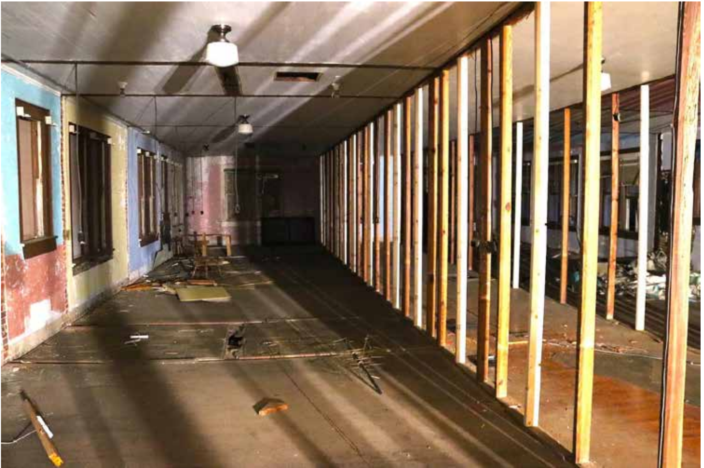
Interior Lamar Hotel rooms are defined by the different paint colors on their respective walls, scars on the floor, and unpainted ceiling strips. The skinny room with the red and blue exterior wall on the far left was a pair of bathrooms. Windows opened onto a lightwell that has since been roofed over. The remaining wall studs mark the wing's central hallway. (Photo by Brian Hughes)
