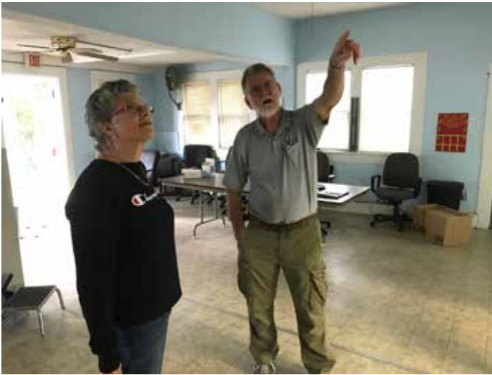
Tanya Nunes, the great-great-granddaughter of Lorenza and Laura Bush, examines renovation details with Rick Rausch of Triple R Construction who is overseeing renovation of the 1926 Bush House.
