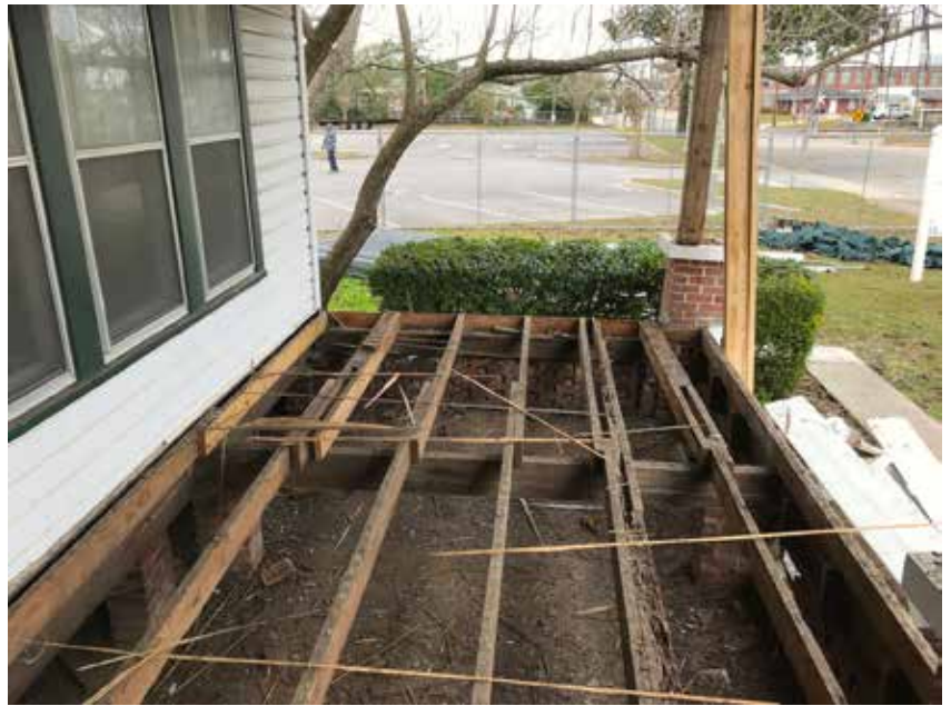
The north front porch decking is removed for replacement and the four front 6"x6" columns will be replaced. The actual columns were encased inside a painted wooden box made to look like concrete columns.
