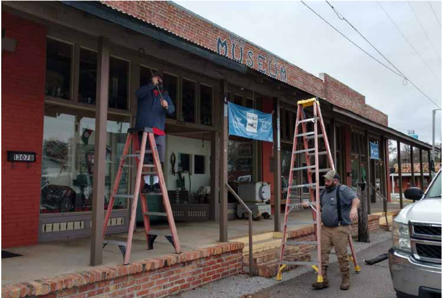
Workers from Hub City Glass repair fire damage along the the Museum's porch December 9, 2021, from the May RV fire (above).
