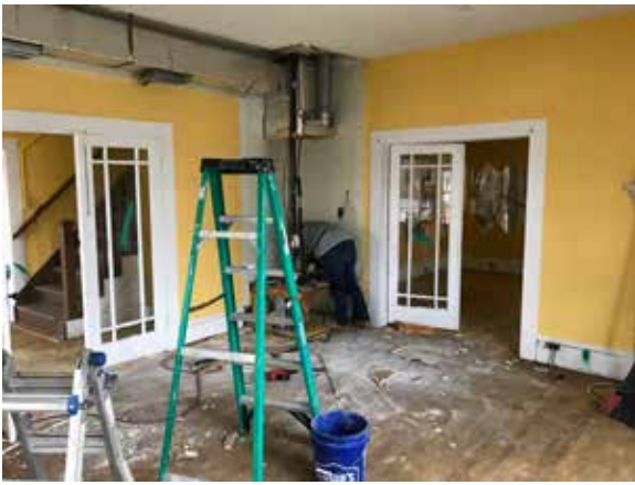
A worker removes a heating unit from the corner of the Bush House front parlor, making the room seem larger. The ducts above him were also removed.
