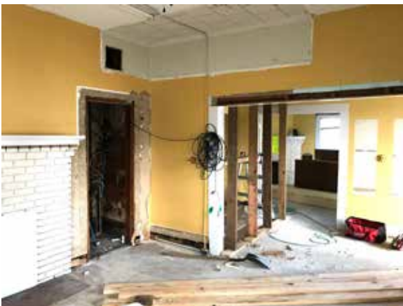
A formerly enclosed doorway into the large back room is revealed during renovation. Ductwork has been removed from the ceiling, and the removal of a fascia above the opening to the room shows what may have been the header of a single door. Pulling up the gray commercial carpeting revealed heart pine floors throughout much of the house. These will be sanded and refinished.
